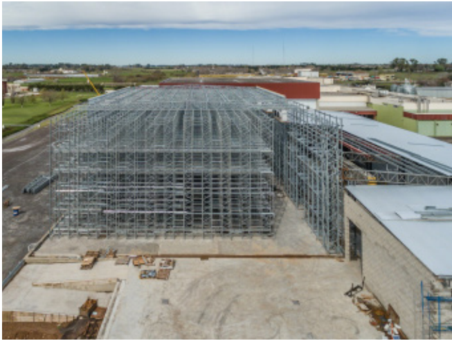
A clad-rack warehouse with a frozen product chamber.
